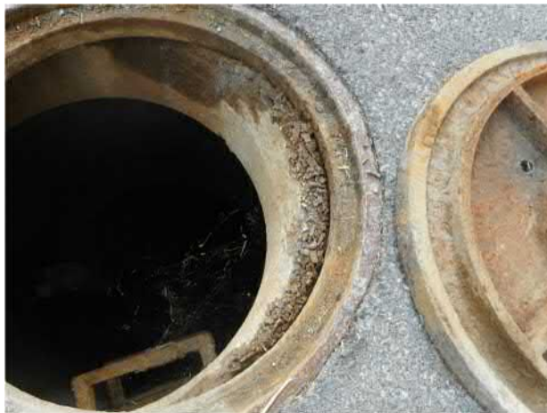
Manhole 5-27: Offset Frame
