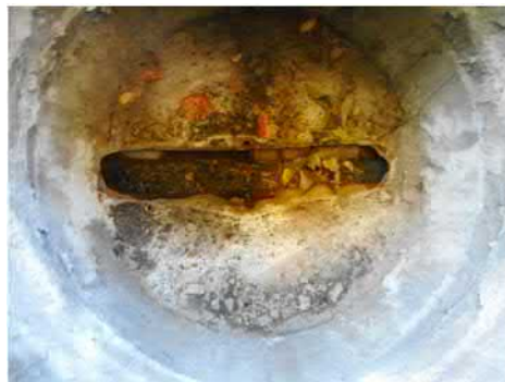
Manhole 2-14: Deposits on Bench/Channel
