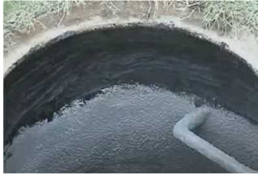
Manhole Chimney Seal
