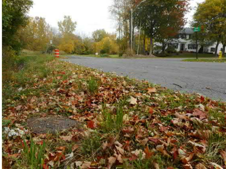
Manhole 7-13: Low Lying Manhole Cover
